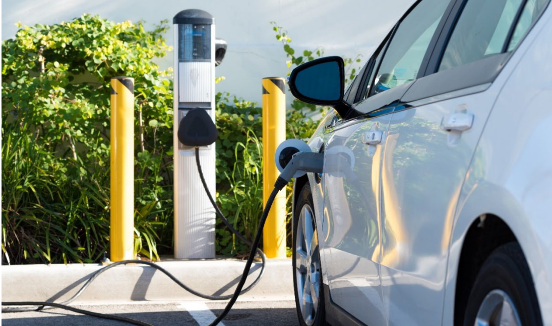
Figure 8. Electric car charging.
