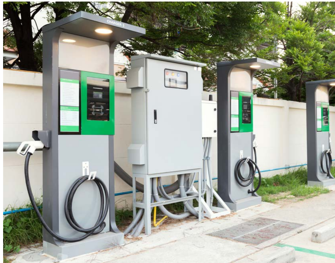
An electric car charging station ready for use.
